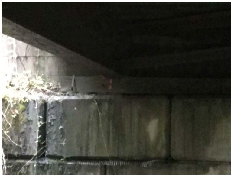
Upstream left bank shimmed
