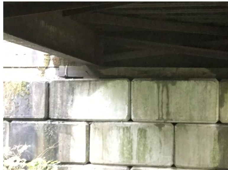
Downstream right bank shim
